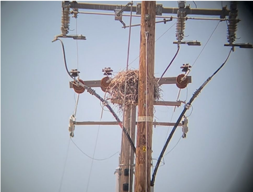
Photograph 4: East Corral Hollow Road, showing nest present on utility pole along roadside in BSA.
