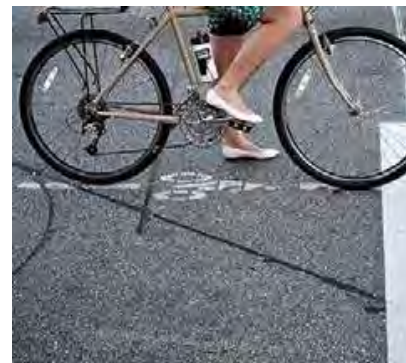
Bicycle Detection Loop in Long Beach, CA – Source: City of Long Beach
