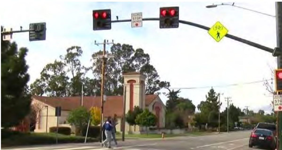
Pedestrian Hybrid Beacon in San Luis Obispo, CA – Source: SLO Chambers
